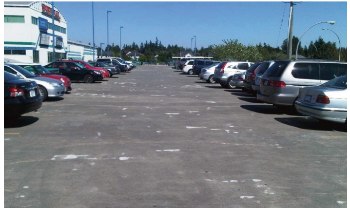
Sportsplex Arena parking shows signs of deterioration.
